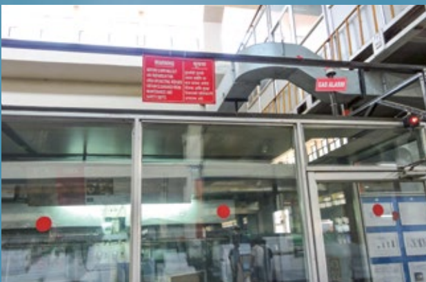
Figure 14: Ventilation system and gas alarm of test performance lab
