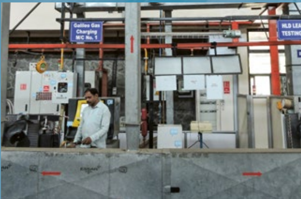
Figure 12: Ventilation system of refrigerant gas charging station
