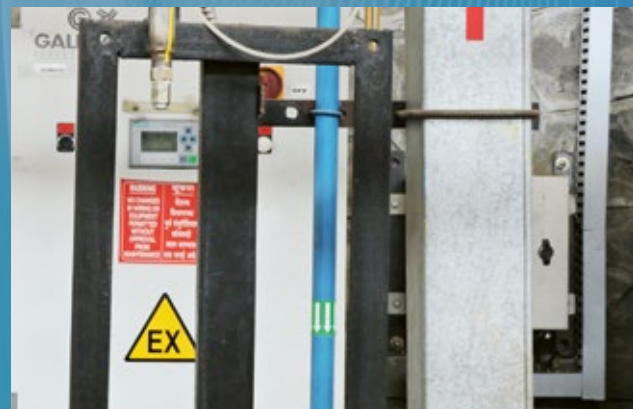
Figure 15: ATEX certified control panel
