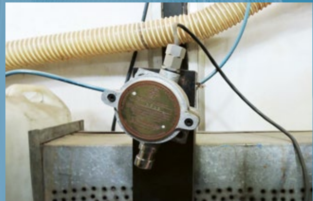
Figure 13: Gas detector at gas charging station
